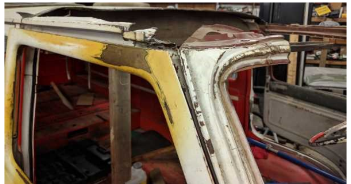
Pass. side front with alignment references and identified issues.
