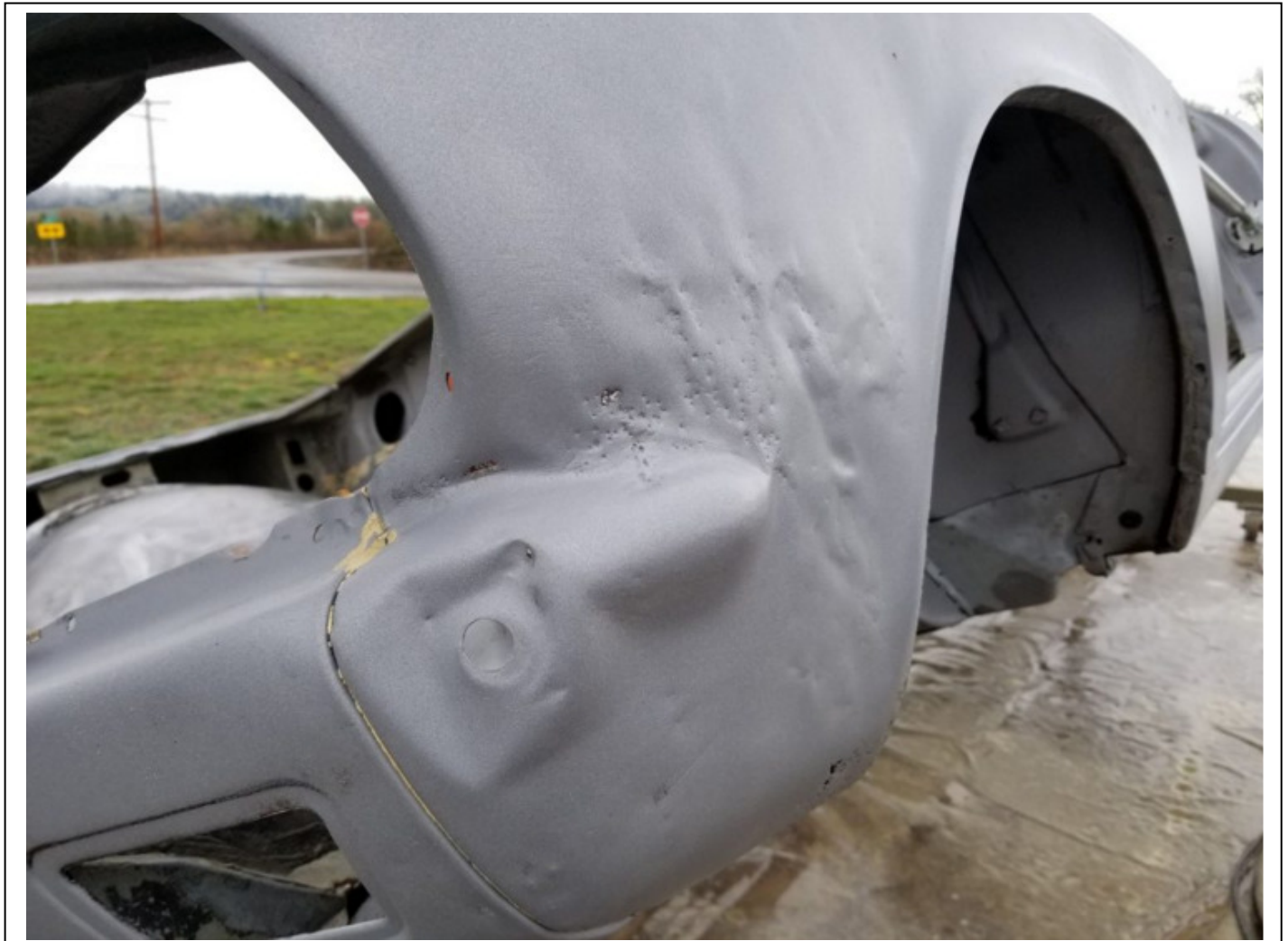
Evidence of a past collision repair, likely done to a price instead of a standard.
