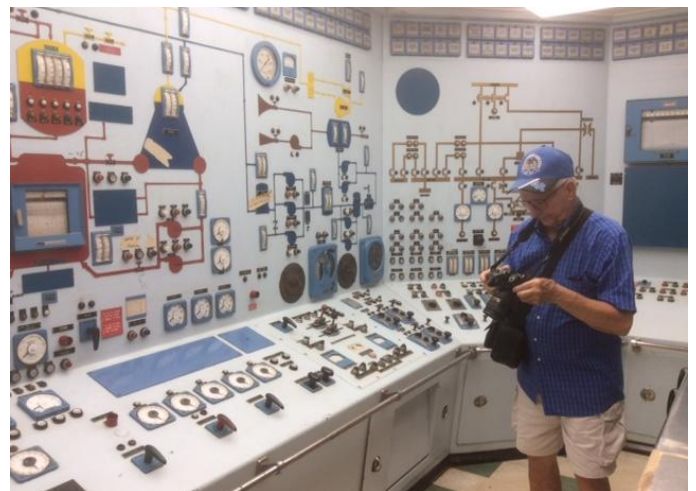
Reactor Control Room
